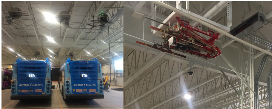
Figure 21 - Cable Reel (Left) and Overhead Pantograph (Right)
